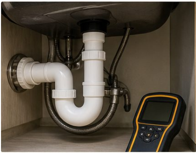
Basin | Photo 1 Vanity pipework - illustrative sample image, not evidence of a diagnosed leak
